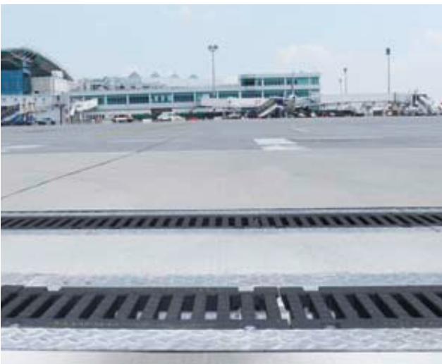
Reliable drainage of huge areas
